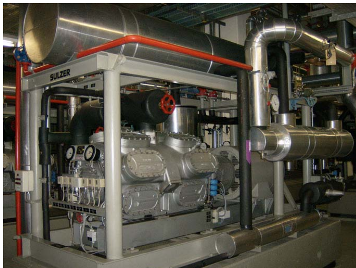
Figure 9: One of the four 440 kW heat pumps of the Lucerne railway station (1984) [Axima, CH-6010 Kriens]
