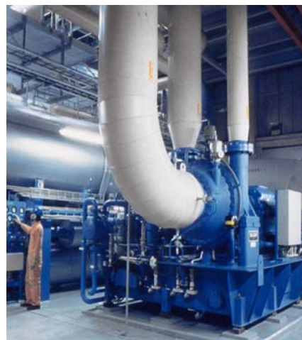
Figure 11: One of six 30 MW Sulzer heat pumps at the Stockholm district heating (1985) [www.friotherm.ch]
