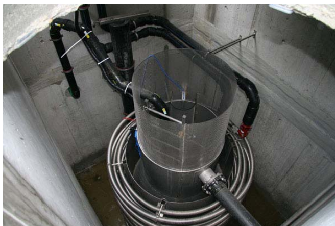
Figure 13: FEKA-tank for the heat recovery from raw sewage [Kalberer, FEKA-Energiesysteme, CH-7310 Bad-Ragaz]
